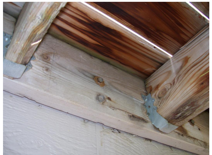
Install proper flashing at the deck ledger/wall interface to prevent moisture damage.
