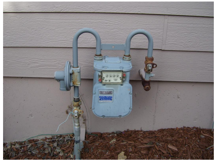
The main gas shutoff
