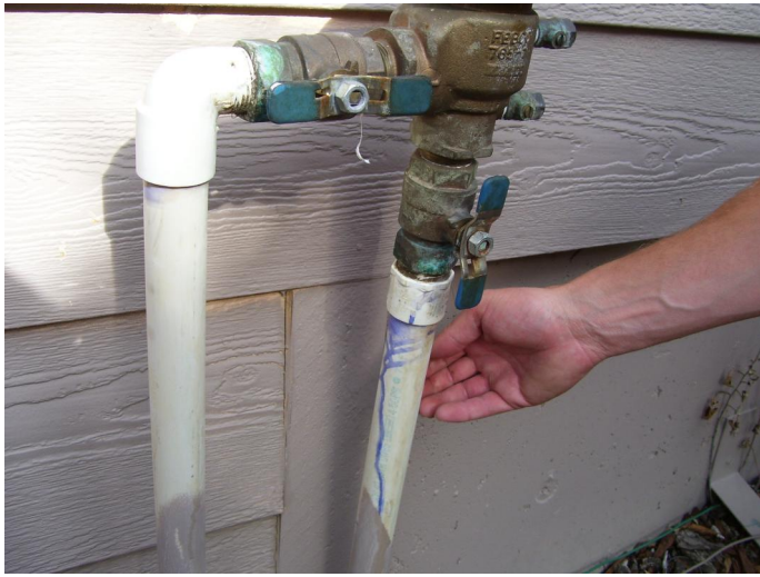
Repair the active leak at the exterior sprinkler backflow device
