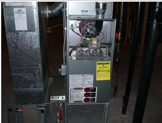
The furnace appears serviceable at this time
