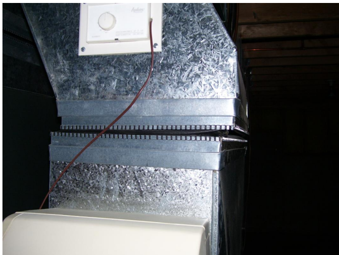
Install an expandable boot in this basement furnace truck line per current standards.
