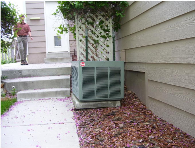
Monitor this east side A/C compressor for further settling.
