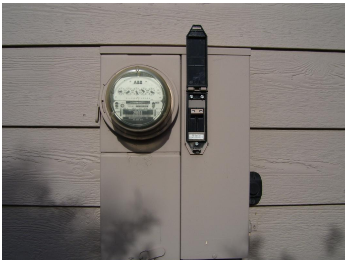
The main electrical disconnect
