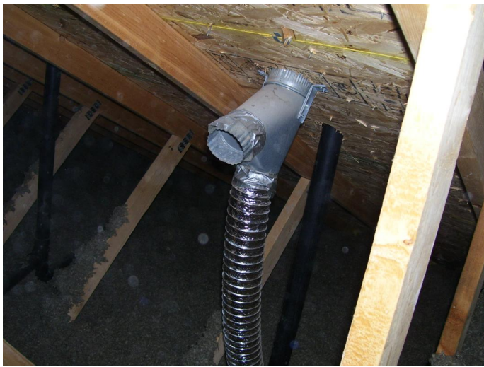
Re-connect this bath fan exhaust duct in the attic space
