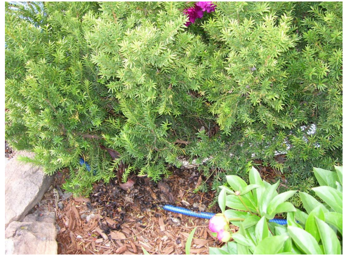
Clean out the gutter downspout extensions for proper roof drainage away from foundation.
