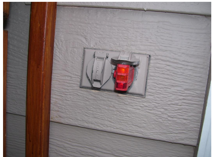
Have an electrician correct the reversed polarity at the rear deck outlet
