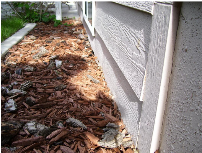
Replace the moisture damaged bottom course of masonite siding at the north exterior.
