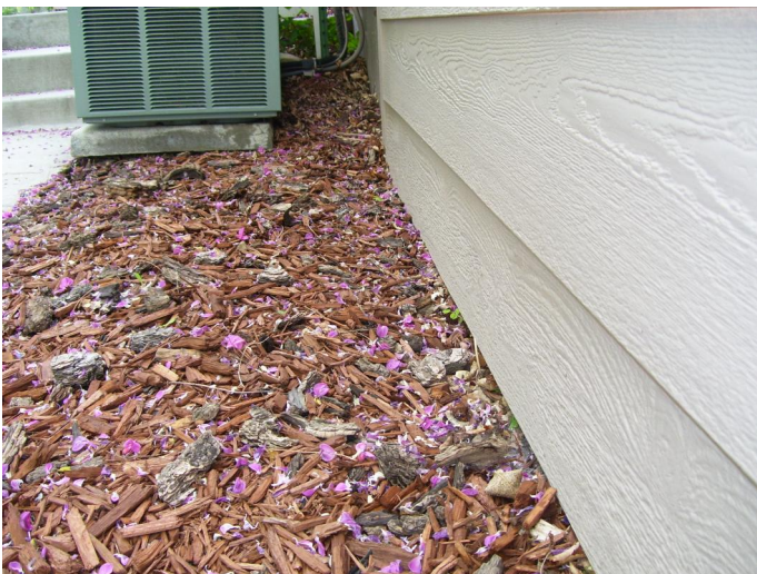
Add fill dirt as needed to create a positive slope away from foundation.
