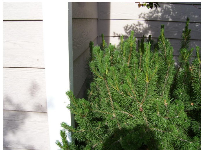
Cut back plants in contact with fibrous siding.
